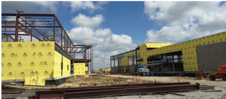
SW MS – Exterior Sheathing/Wall Erection – View towards Area C (Left) to Area E (Right)
